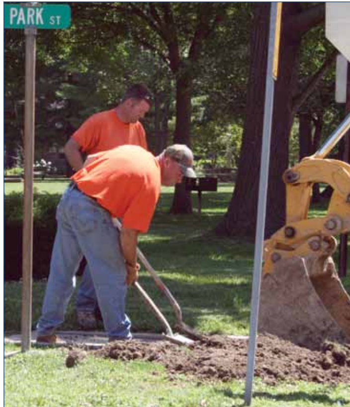
City workers take proper precautions while repairing a water line near Bliss Park.
