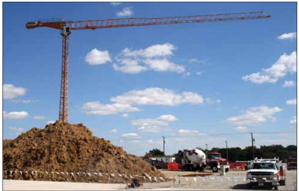
Construction continues on the new corporate headquarters for Midland States Bank. Construction is expected to be completed by Fall 2011.
