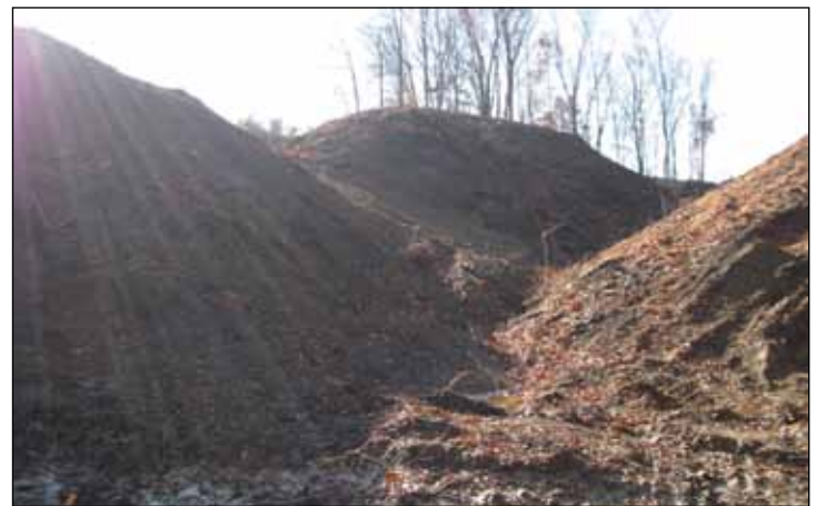
Dirt work has begun on the final leg of Outer Belt West, which will connect Ford Avenue to the existing roadway.
